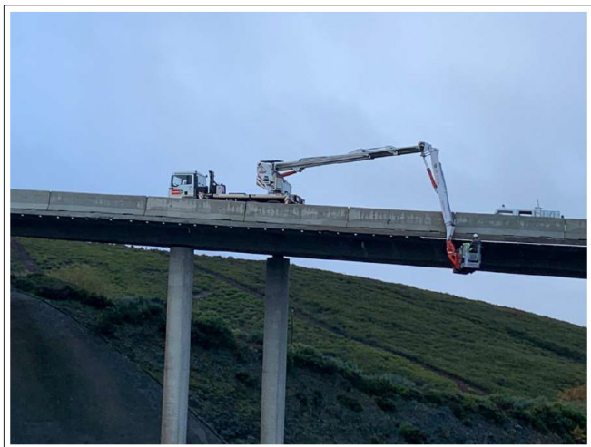
Figure 22: Main Inspection Under the Deck of a Viaduct that Crosses the Rías Bajas Highway (A-52), in the Municipality of A Gudiña, in the Province of Ourense, in Spain (author's Photograph)
