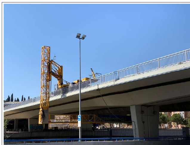
Figure 21: Main Inspection on the San Isidro Bridge, in Madrid, using Specific Equipment to Facilitate Operator Access to the Underside of the Deck (author's Photograph)
