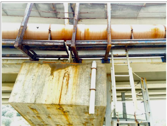
Figure 12: General View of the Shaft of One of the Piers, Where Corrosion Phenomena can be Seen that Affect different Constituent Materials of the Structure (Photograph Taken with the Anafi Parrot Drone).
