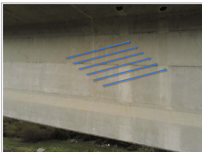
Figure 20: Diagonal Crack in the Beam Web, Caused Presumably by a Shear Stress (Photograph Taken with an Anafi Parrot Drone).
