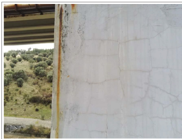
Figure 15: Fissuring on the Map that Denotes Injuries Due to Plastic Shrinkage, Hydration Heat or Suffocation (Photograph Taken with the Anafi Parrot Drone)
