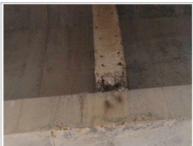
Figure 11: Detail of the Element in Figure 10, Where a Chipping and the Consequent Corrosion of the Exposed armor Can be Seen (Photograph Taken with the Anafi Parrot Drone).
