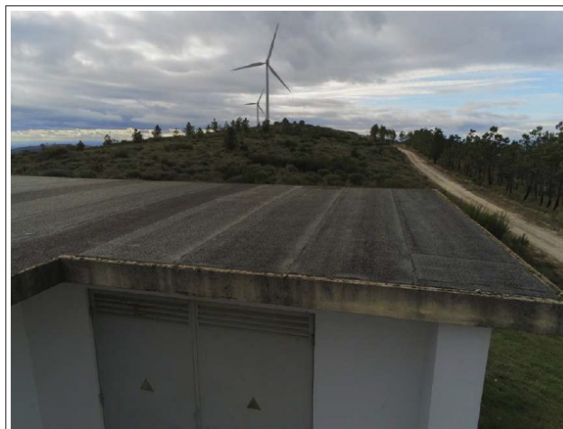
Figure 24: Transformation and Control Center Roof Inspection in a Wind Farm Located in Torre de Moncorvo, Bragança (Portugal) for the Location of Deficiencies Causing the Humidity Recorded Inside (Photograph Taken by the Author with an Anafi Parrot Drone).
