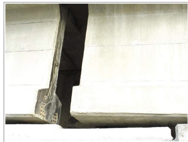
Figure 18: Detail of One of the Beams, Where the Chipping of the End of the Wing Area can be Seen, Leaving the Prestressing Tendons Exposed (Photograph Taken with the Anafi Parrot Drone).
