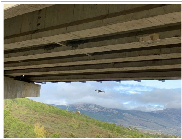
Figure 8: Anafi Drone Flying Over Under the Beams that Support the Deck in the First Span (the Nearest to Madrid) to Recognize the Constituent Elements of the Viaduct (author's Photograph)
