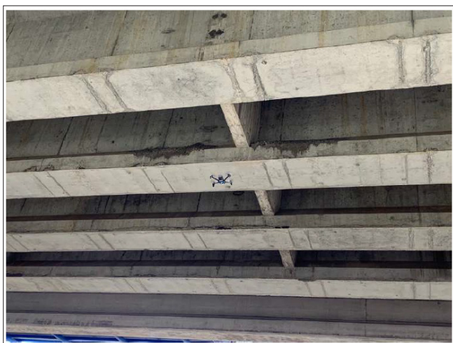
Figure 16: View of the Drone Approaching the Space between Two Beams, for the Analysis of the Non-Visible Faces of the Beams (author's Photograph)
