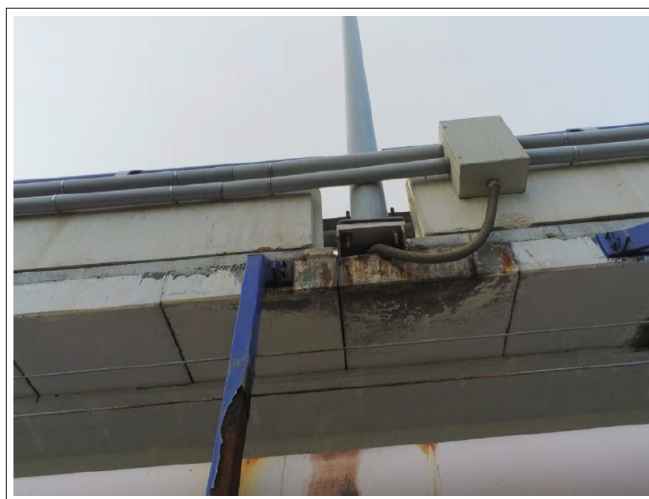
Figure 9: Signs of corrosion in concrete and metallic elements. Note also the poor support of the staff, as two of the four bolts at the rear cantiléver (photograph taken with the Anafi Parrot drone).
