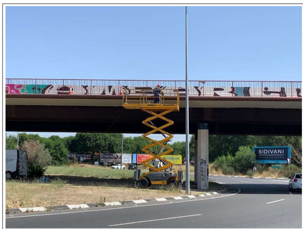
Figure 1: Operations within A Special Inspection Carried Out in A Mixed Structure (Concrete and steel) using A Personnel Lifting Platform (author's Photograph)
