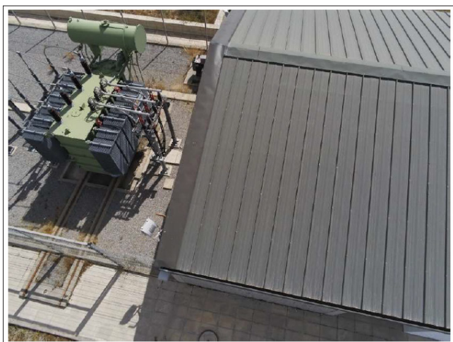
Figure 26: Electrical Substation Roof Inspection in Cinfães, Viseu (Portugal) to Verify Damage after a Heavy Hailstorm (Photograph Taken by the Author with an Anafi Parrot Drone).
