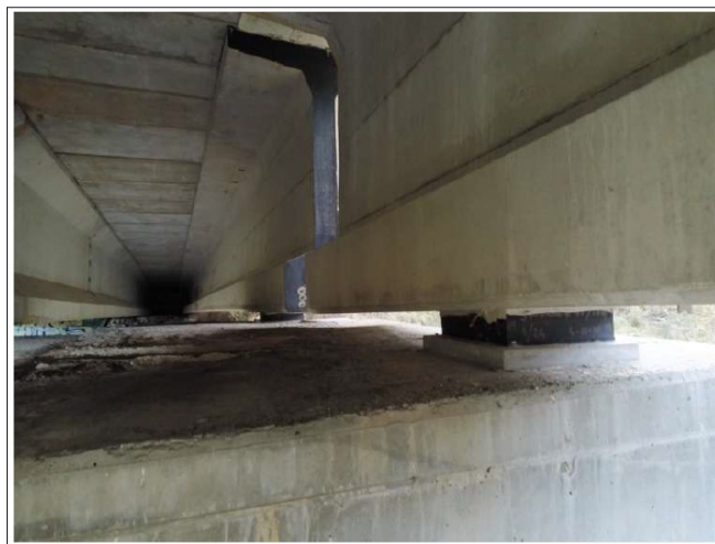
Figure 17: View Under the Deck of the Structure Towards Madrid, in Which it is Observed, in Addition to the Interior Faces of the Prefabricated Beams and the Precast Slabs, the Support Devices Under Some of the Beams (photograph Taken with an Anafi Parrot Drone)
