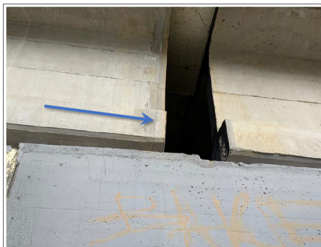
Figure 19: Two Beams Detail, where two Chips can be Seen at the Ends of the Wing Area, Leaving, as seen in the Beam on the right, the Prestressing Tendons Uncovered (Photograph Taken with the Anafi Parrot Drone).
