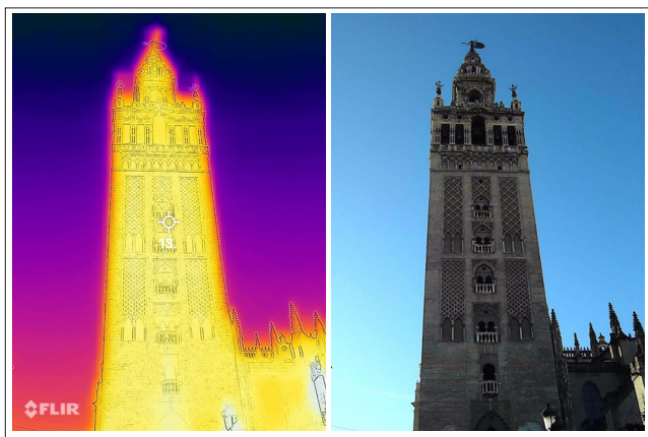
Figure 9: Thermographic Analysis of the North Facade of the Giralda Bell Tower (Photographs by the Author).
