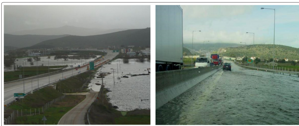
Figure 1: Plain flood in Epirus, Egnatia Motorway inundated (2010): Low embankment in flood-prone area
