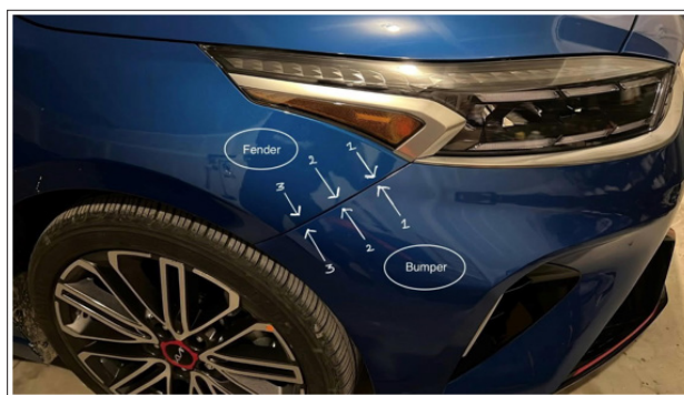
Figure 2: Gap Present between Bumper and Fender on Right-Hand Side
