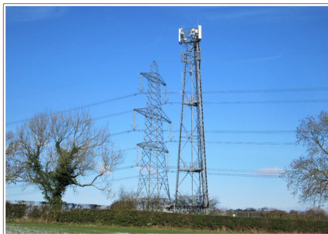
High voltage powerlines with a mast for microwave signals. A formidable combination [6]. Easingwold, North Yorkshire, England. Photo by author.
