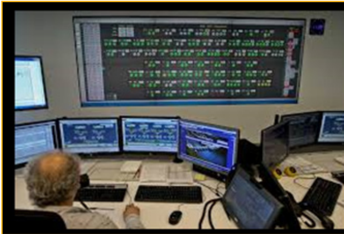
Figure 4: Dispatch Center of EDP Renewables [14].
